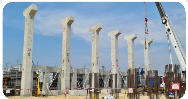
● Pipe Rack Freeport Smelter Gresik
